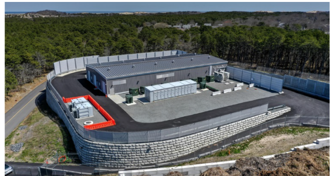
Fig. 2. Provincetown BESS plant
