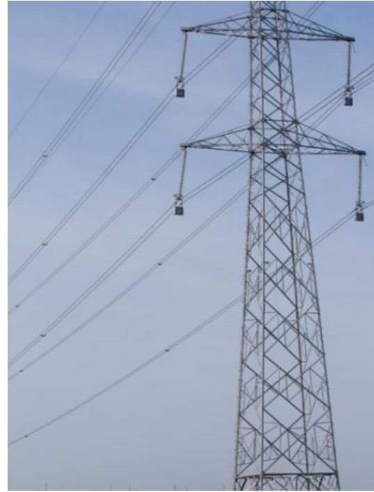
Better power system stability
