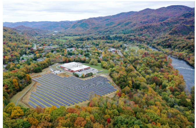
Fig. 2 Hot Springs Battery Energy Storage System (BESS)
