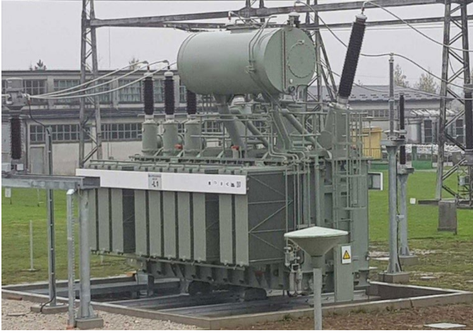
Fig. 3. An oil-immersed iron-core shunt reactor.
