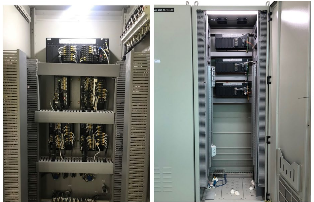
Figure 9: Protection panel at a typical conventional substation vs protection panel at 110KV Nghi Son Digital substation
