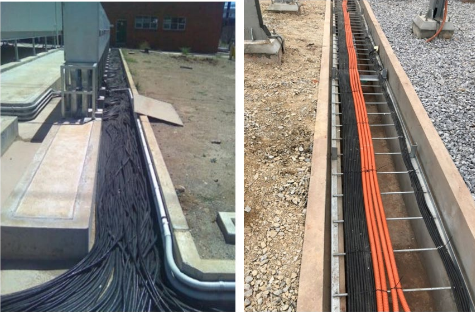
Figure 8: Outdoor cable at a typical conventional substation vs Outdoor cable at 110KV Nghi Son Digital substation
