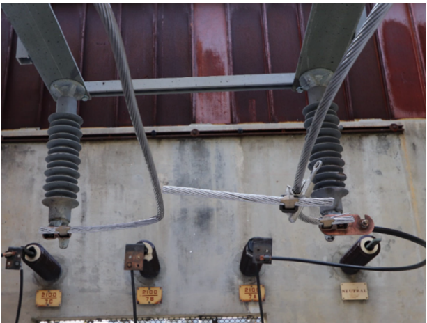
Figure 3. Pigtail conductor configuration in "Cage" test.
