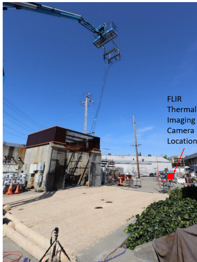
Figure 5. Lift test environment, showing location of FLIR Camera.
