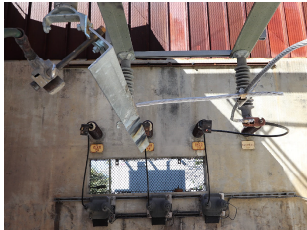
Figure 4. Pigtail conductor configuration in "Cage" test, testing against a leg simulating a steel transmission line component.
