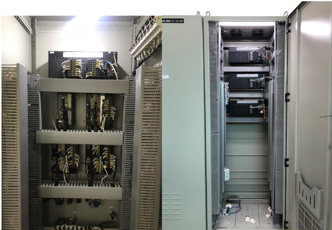
Figure 9: Protection panel at a typical conventional substation vs protection panel at 110KV Nghi Son digital substation
