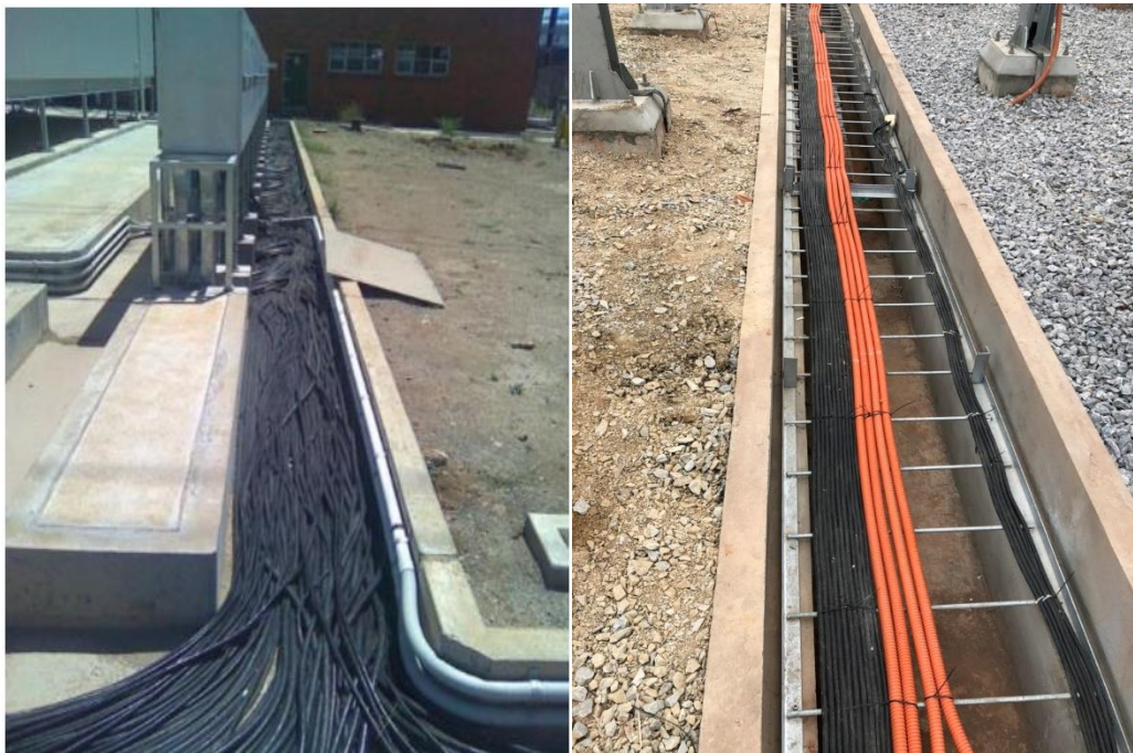
Figure 8: Outdoor cable at a typical conventional substation vs outdoor cable at 110KV Nghi Son digital substation
