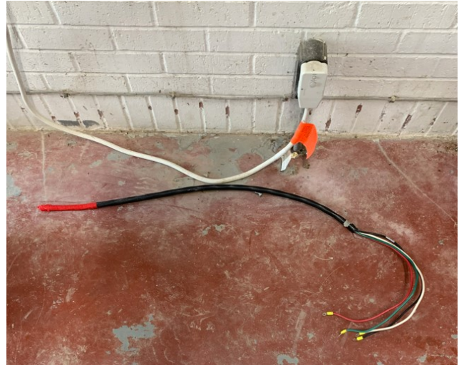
Fig. 3a. 4-wire bundle cut and left behind in the substation house
