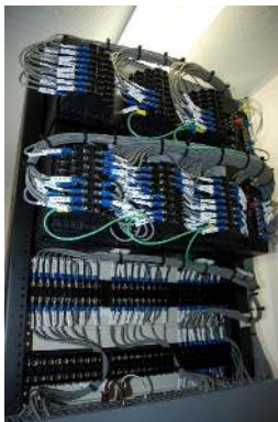
Figure 4: Multi application copper wiring
