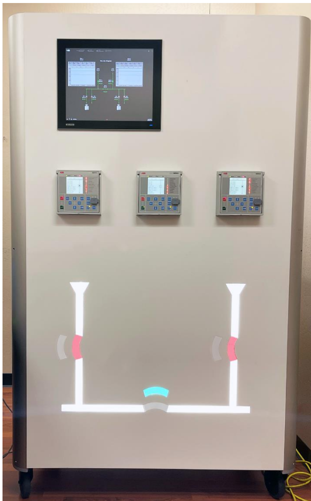
Figure 11 The demo unit in Main-Tie-Main arrangement with illuminated schematic and breaker position (red close, green open), performing a simulation of loss of power on one of the sources, front view
