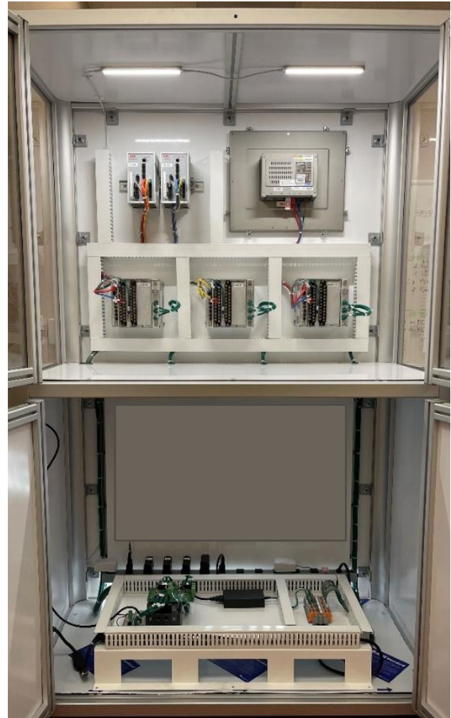
Figure 12 The rear view of the demo unit, on top: relays, HMI and network switches, bottom: signal generator
