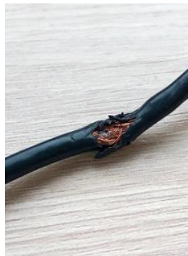
DC control system faults
