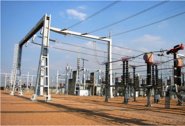
Substation A, owned by company X
