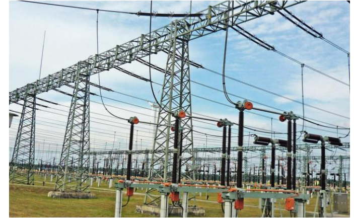
Substation B, owned by company Y
