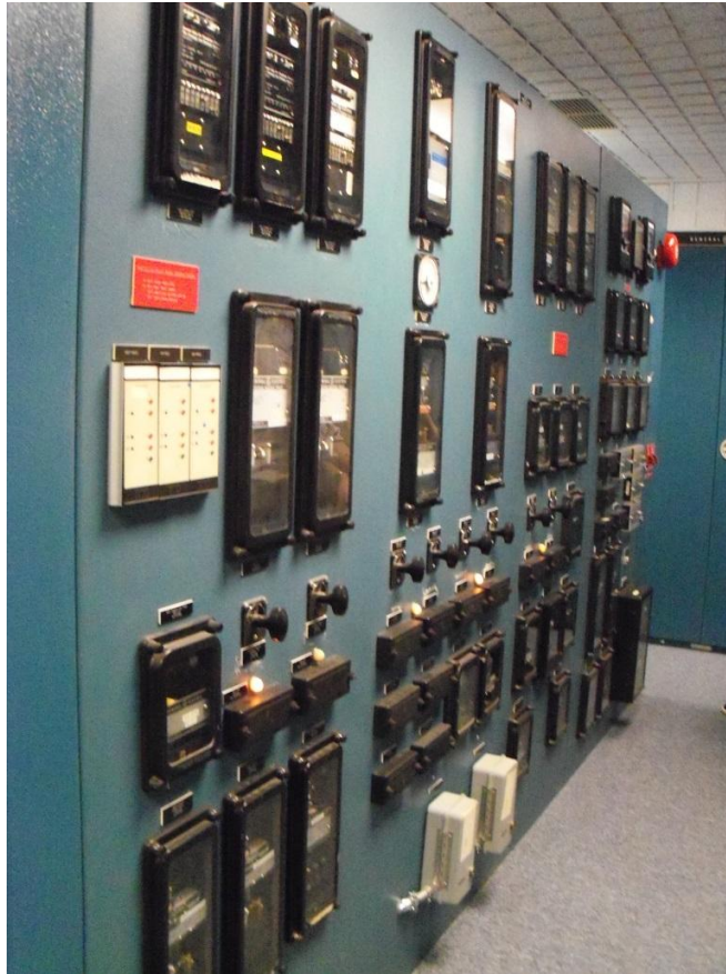
Picture 1: Existing generator and transformer protection panels
