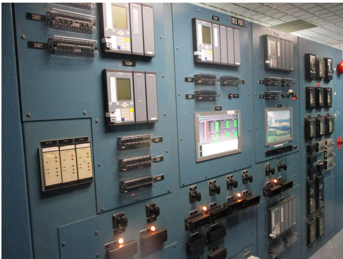
Picture 2: Upgraded generator and transformer protection panels
