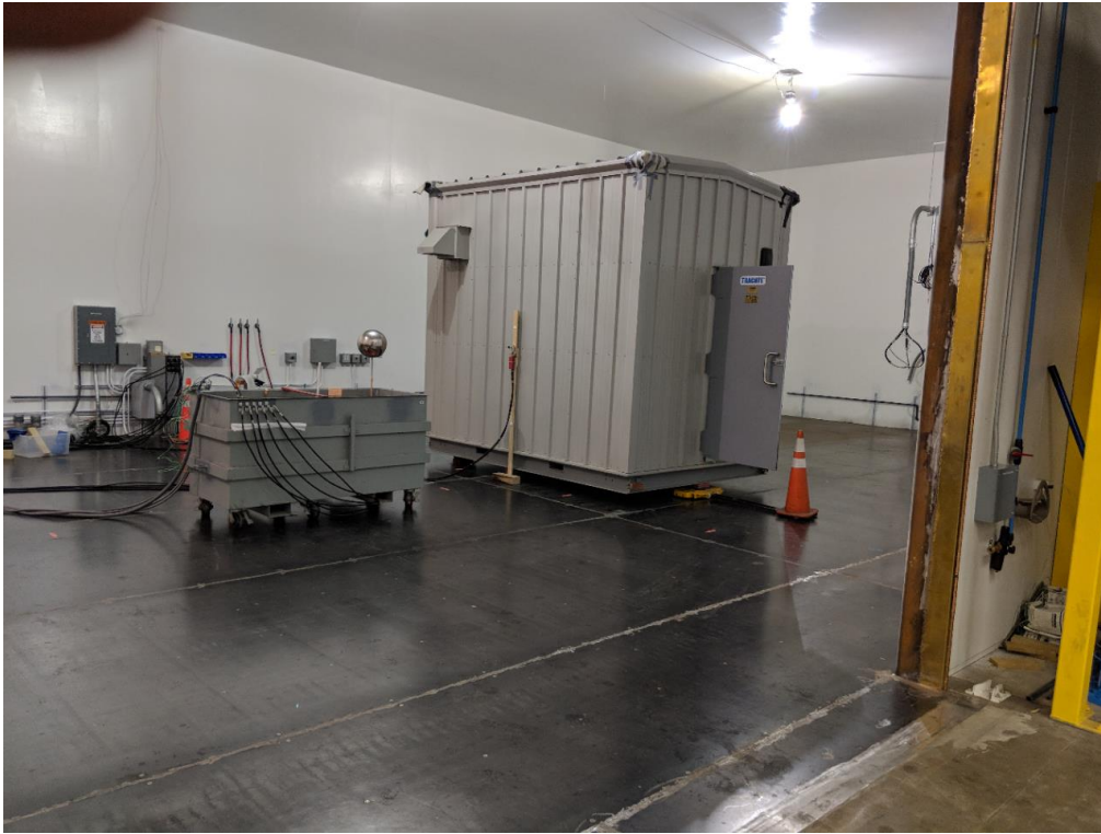
Figure 8 Test Generator and Control House in Test Chamber
