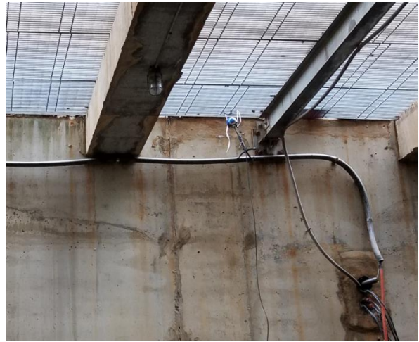
Figure 12: GPS Strapped to the top of the vault for increased signal strength
