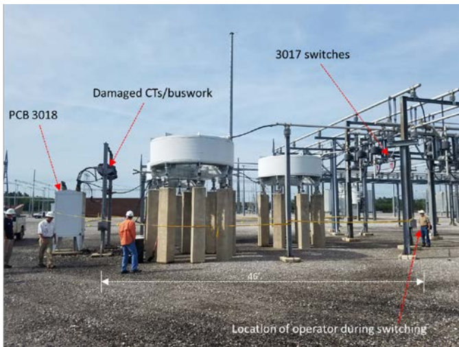
Fig. 12. Side view photo - 3018 shunt reactor, with dimensions
