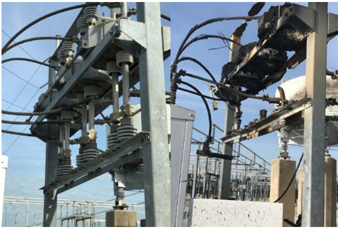
Fig. 8. Good installation vs damaged installation
