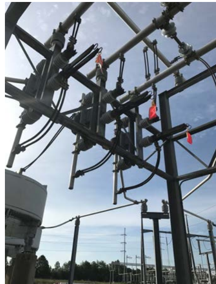
Fig. 16. Dual-blade non-ganged manually operated (via hotstick) single-phase disconnect switch 3017
